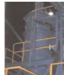
40m 2 Industrial Installation
